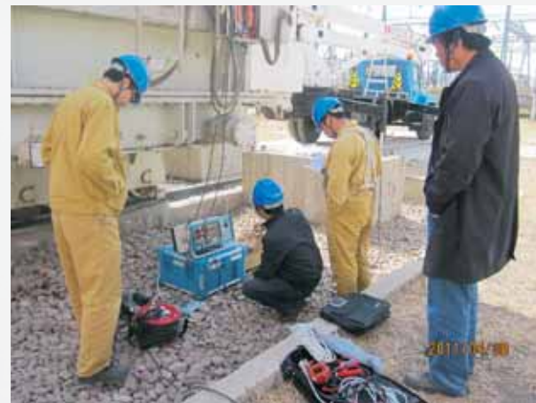
500kV Tranformer Bushing CT
