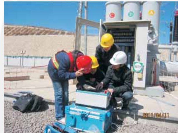
220kV Transmission Line CT
